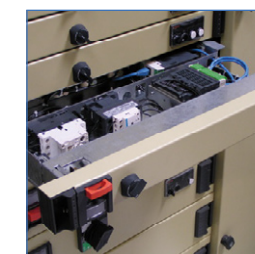
Equipment with TeSys T motor starter
