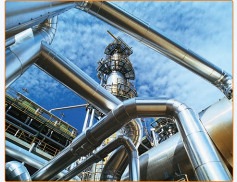
Chemical, Oil and Gas
