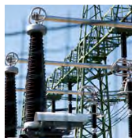
Electrical generation, transmission, distribution, installation & maintenance
